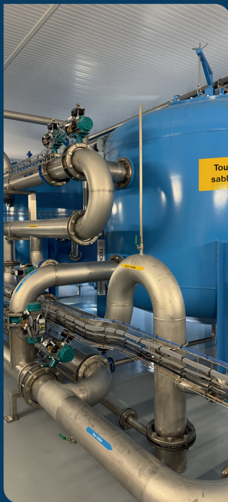
Station de production, Le Jourget, Montcaret.
